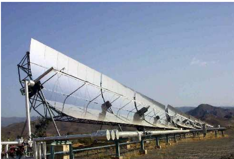
Figure 1. DISS facility at Plataforma Solar de Almería (Southeastern Spain).
